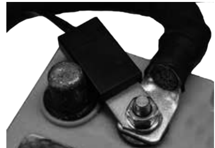
Fig 2.5(b) Temperature Sensor Installation
